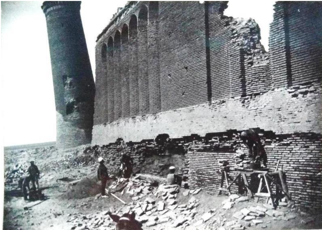
Figure 11. Rabati Malik Caravanserai and Sardoba: Rabati Malik Caravanserai: reinforcement of the foundations of the West wing in 1928. Source: Ministry of Culture of the Republic of Uzbekistan (1928).
