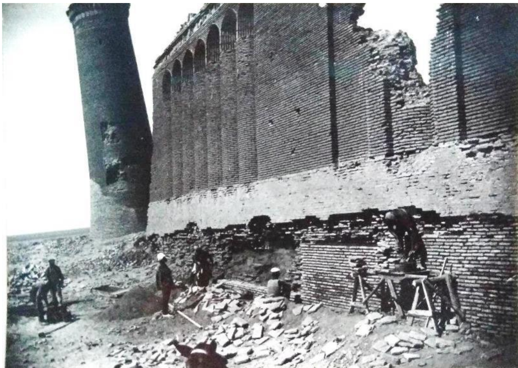
UZ-07. Rabati Malik Caravanserai and Sardoba: Raboti Malik Caravanserai: the repair works in 1937. Source: Ministry of Culture of the Republic of Uzbekistan (1937).
